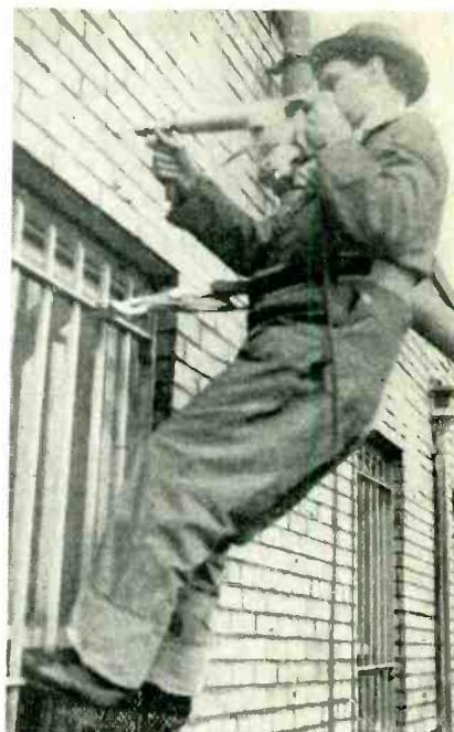
Serviceman working with small electric jack hammer, boring holes in masonry. Note safety belt.
