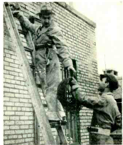
★ Servicemen installing a master antenna system atop an apartment building. Note that they wear safety belts—a worthwhile precaution when working on tall buildings. See article on page 4. (Photo by Austin C. Les-carboursa)
